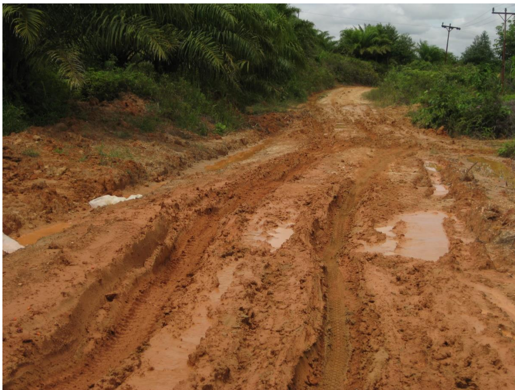
Figure 11: This road is in very poor condition and needs to be improved!
